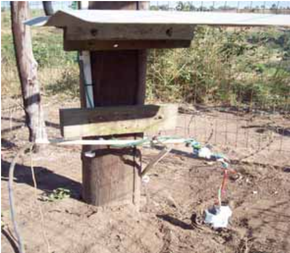
The photo above shows the space where a transformer used to be at the Ndundulu water project in Mthonjaneni Municipality.
