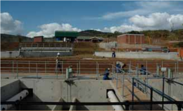
The newly constructed waterworks at Phobane for the Greater Mthonjaneni Water Supply
