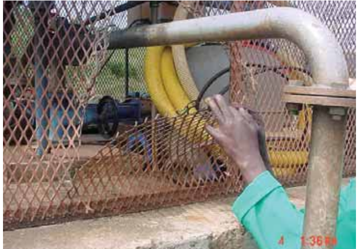
The picture above shows how vandals cut the protective cage to gain access to steal a pump at Zimbidla in Nkandla.
