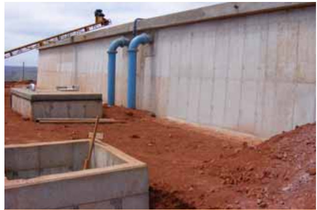
A 2.5 ML reservoir built at Zigagayi as part of the Greater Mthonjaneni Bulk Supply
